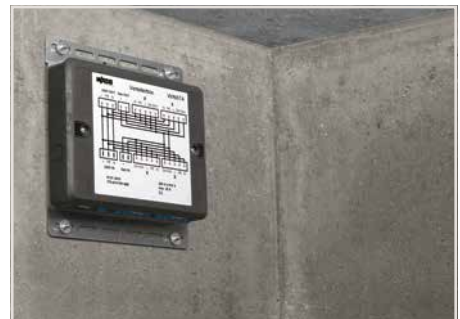
Wall-mounted WINSTA® Distribution Box
